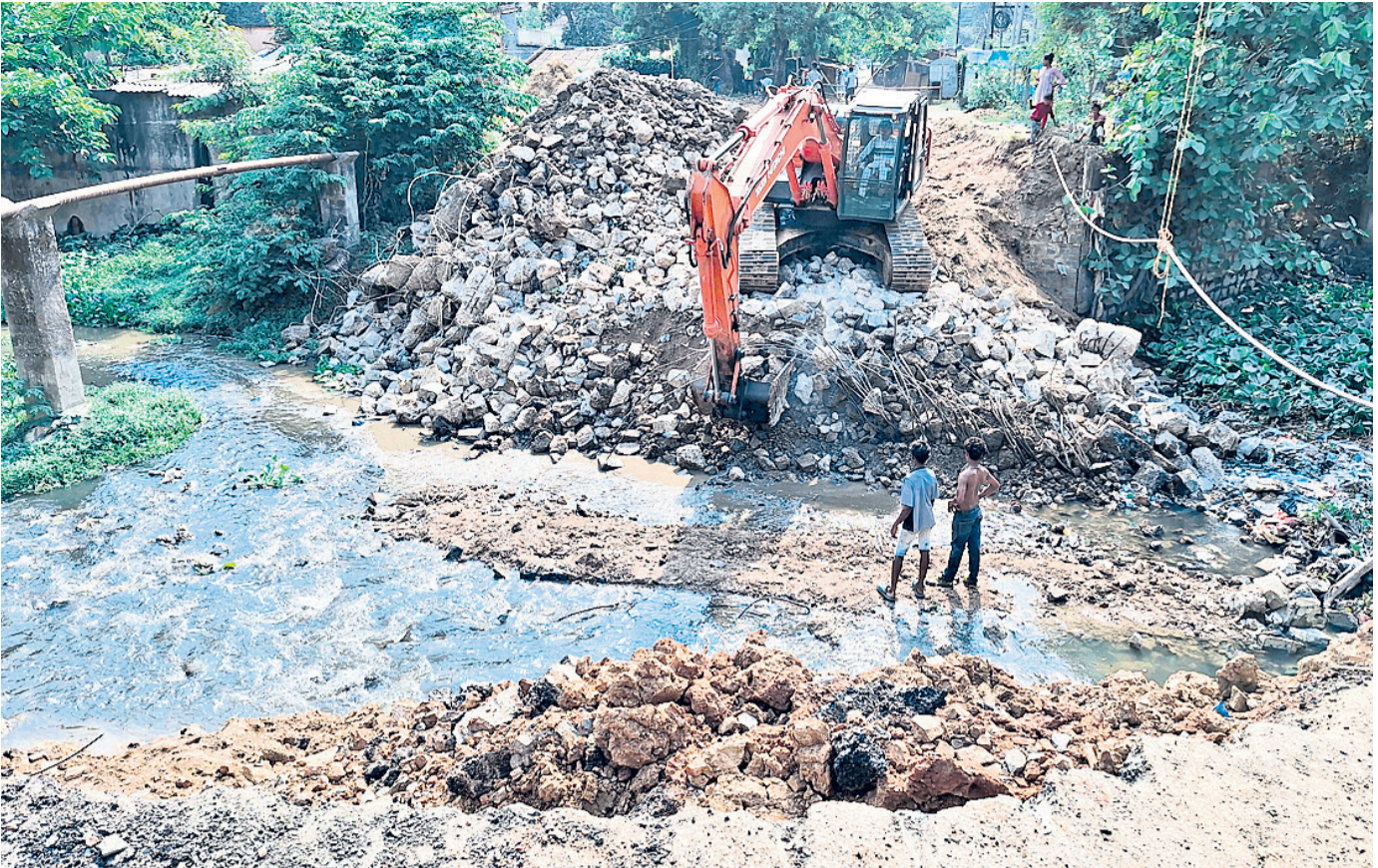
INFRA PUSH: An earthmover dismantling an old bridge connecting Municipality Square to Jail Square in Sambalpur to pave way for construction of a new bridge, Friday
