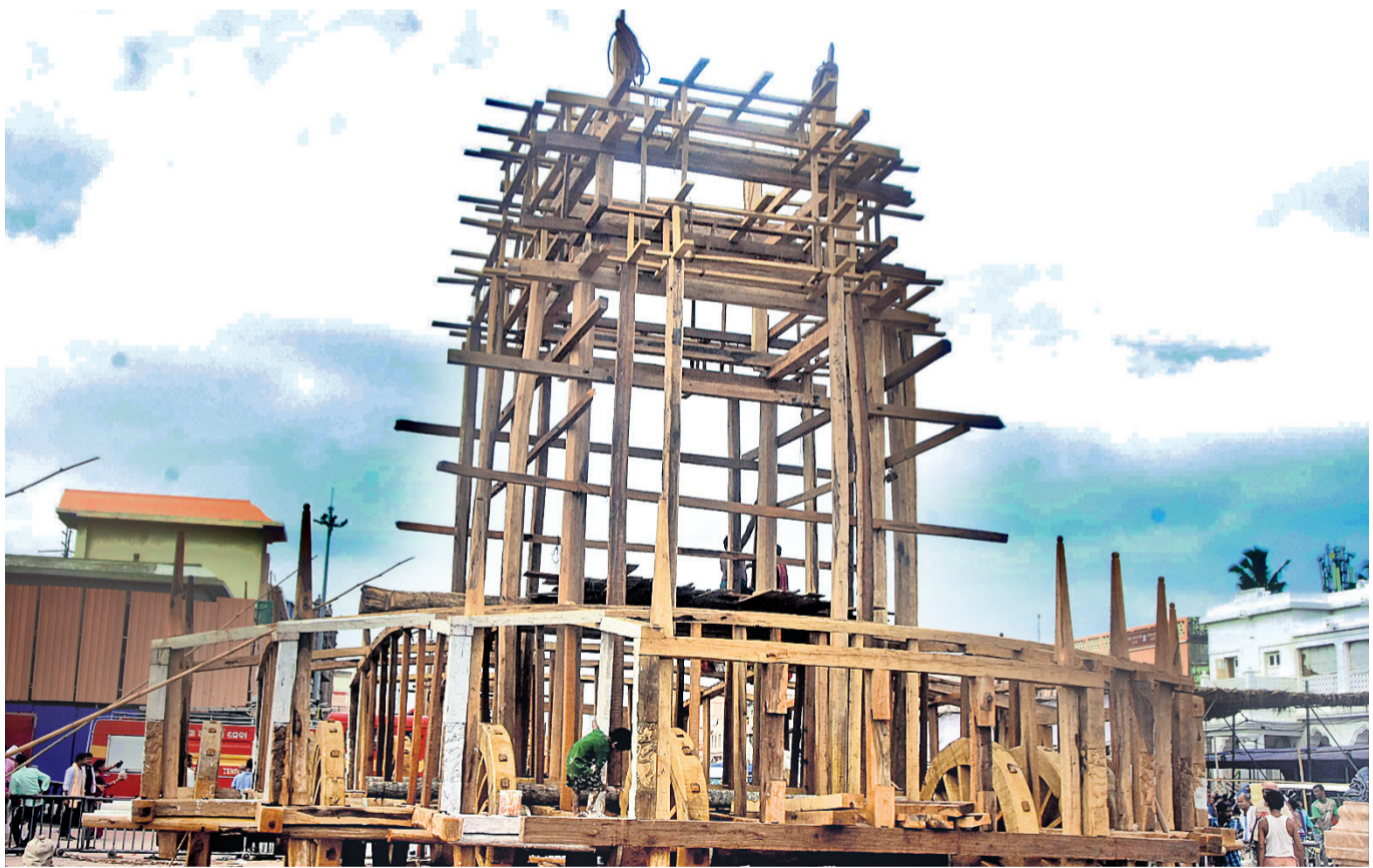
CAR FEST AHEAD: Chariot construction in full swing at Rath Yard in Puri, Sunday
