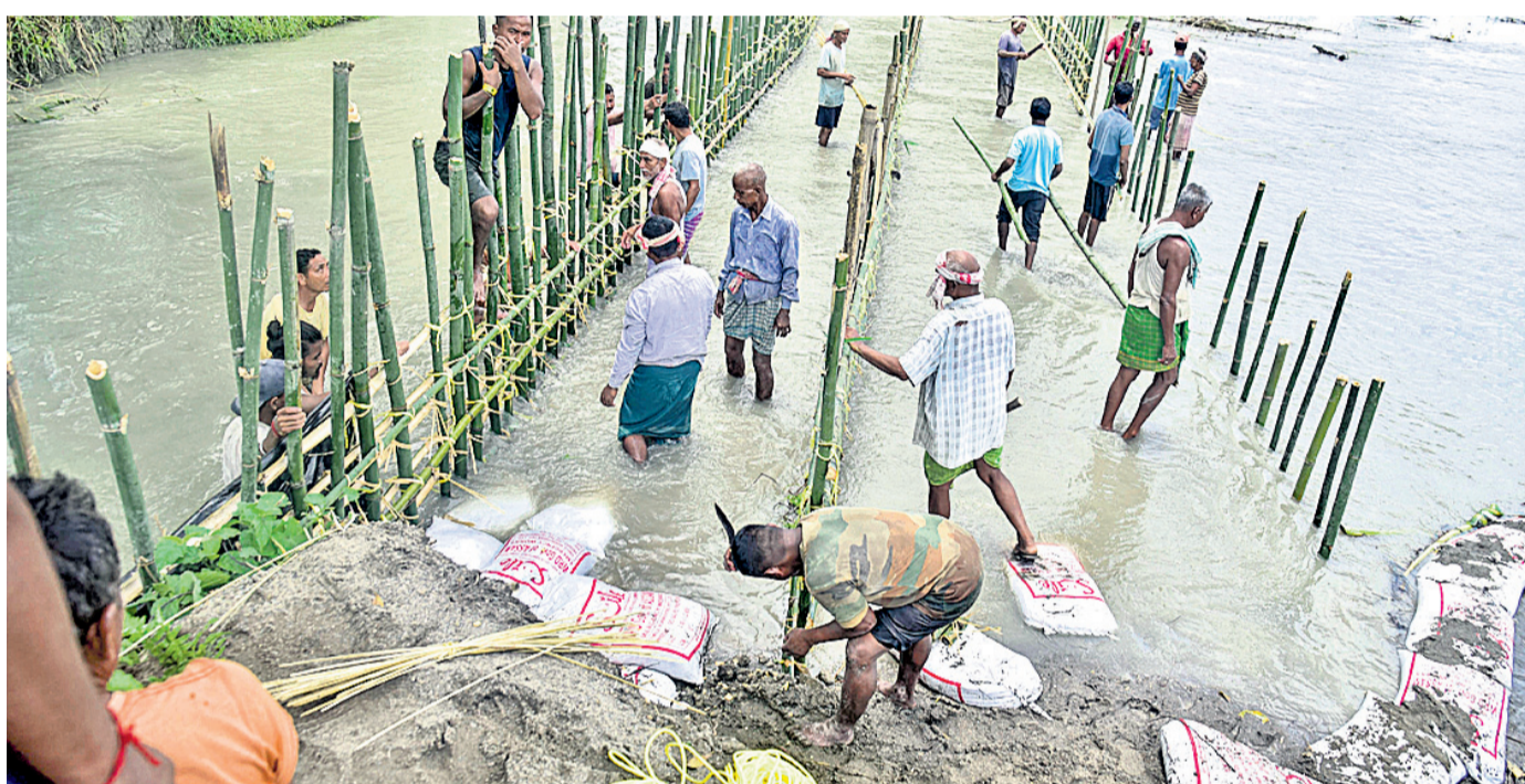
Villagers repair a breach in embankment caused due to floods following rains in Baksa district of Assam, Thursday
