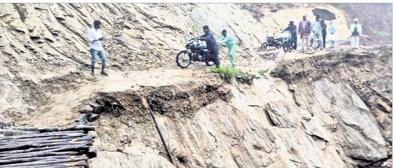
FLIRTING WITH DANGER: Commuters perilously negotiating a stretch on Arangi-Bayapada ghat road under Nakamamudi panchayat of Korukonda block in Malkangiri district, Saturday. Seventeen villages were cut-off from the rest of the world after a bridge was washed away and a major landslide occurred at Tumbapadar. The rainwater flowing down the hill washed away a portion of the ghat road closing the route for traffic (Report P5)
