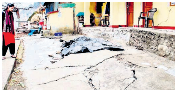
Cracks that appeared in Joshimath last year. FILE PIC/PFI
